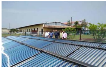
Compound Parabolic Collector field at UCRF Facility
